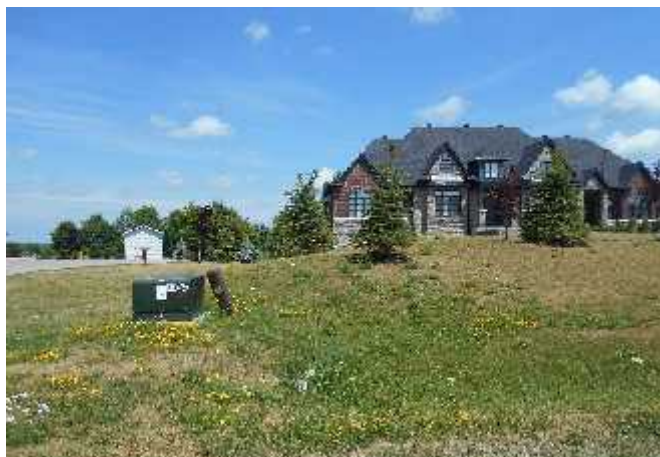
Photograph 21. View of a transformer box along Birdie Smith Court.
